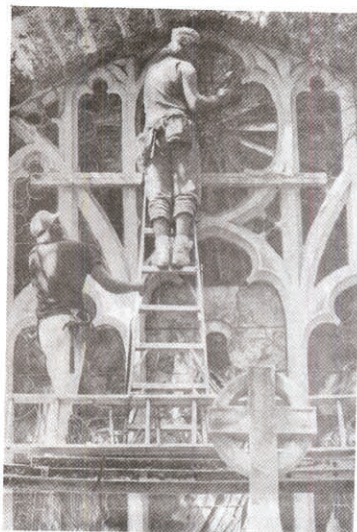
Workers clean a historic stained glass window in Christ Episcopal Church at Franklin Avenue and Castle Place.
